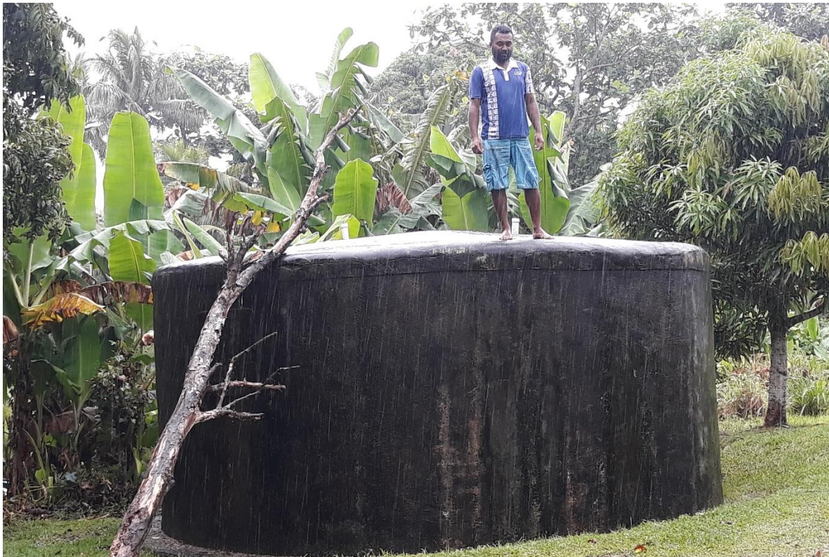
Community water reservoir tank, Daviqele, Fiji (Photo: D. Botero)
